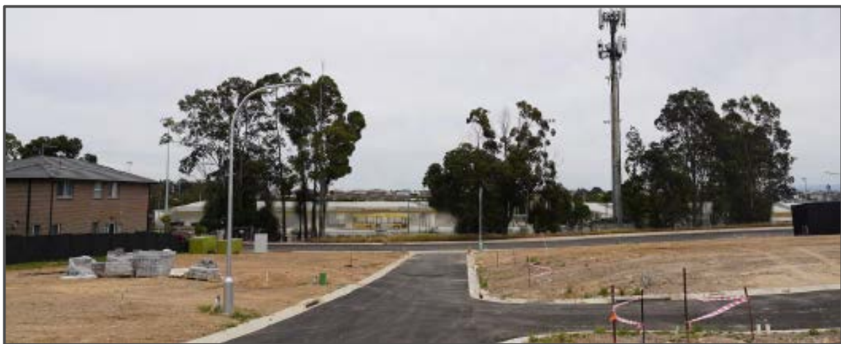
Figure 18 | View 5 of CoE and CF: Newly constructed road off Stone Mason Drive (source: Applicant)
