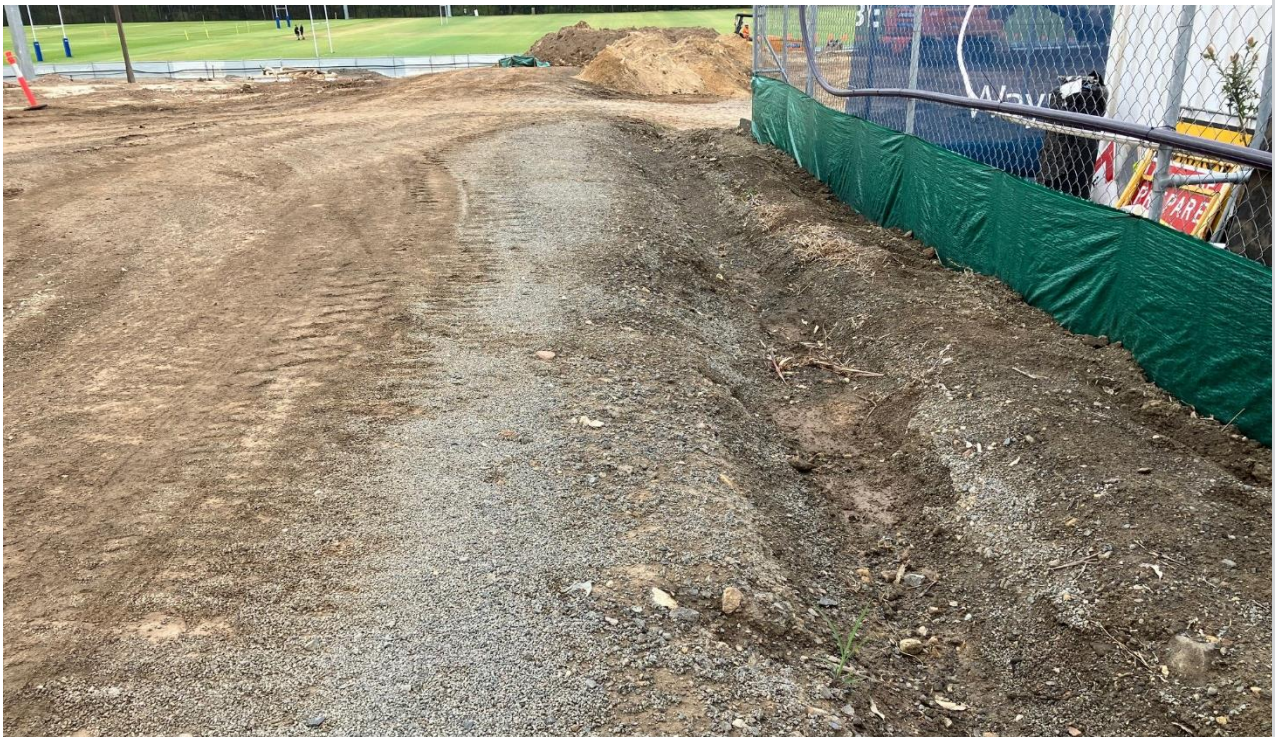
Swales to divert water flow as per erosion and sediment control plan.
