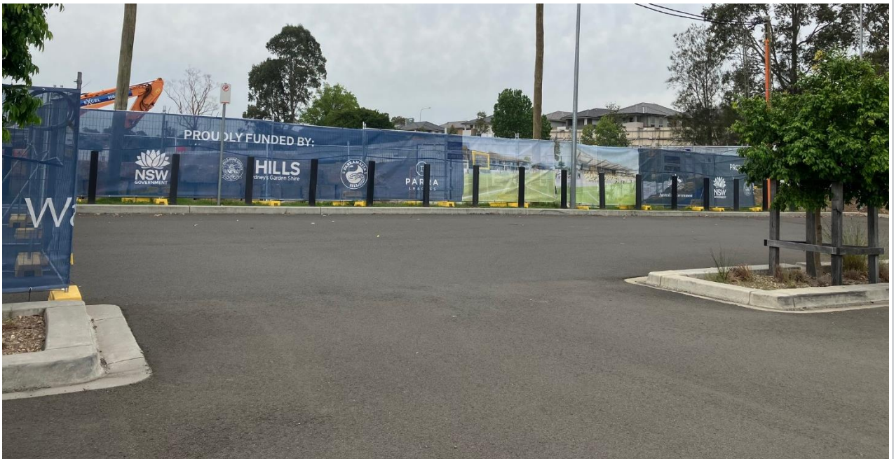
Shade cloth installed around the perimeter of the site. Carpark noted to be clean and clear. Excavator observed within project boundary.
